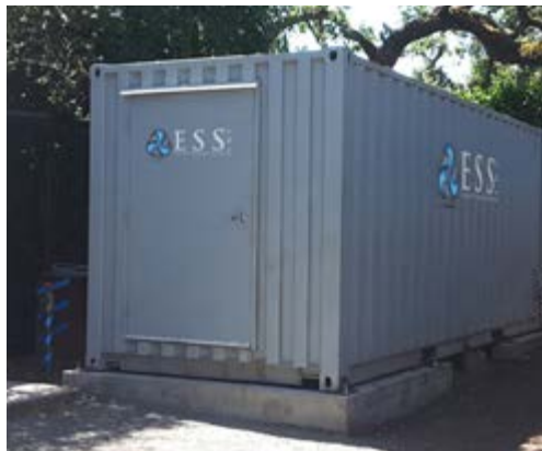
The IFB system installed within an advanced microgrid at Stone Edge Farm.
