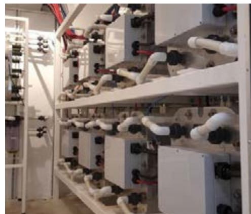
Each Iron Flow Battery and its AC electronic components are housed in a shipping container for transportability and protection from the elements.
