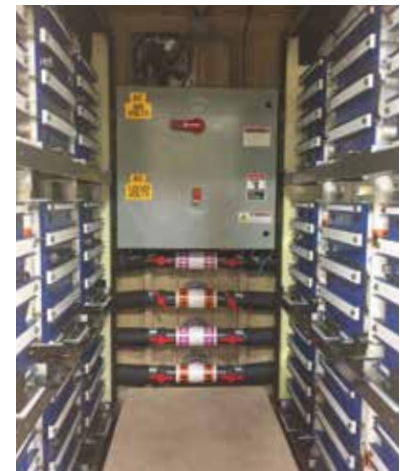
Figure 3: ESS IFB System
